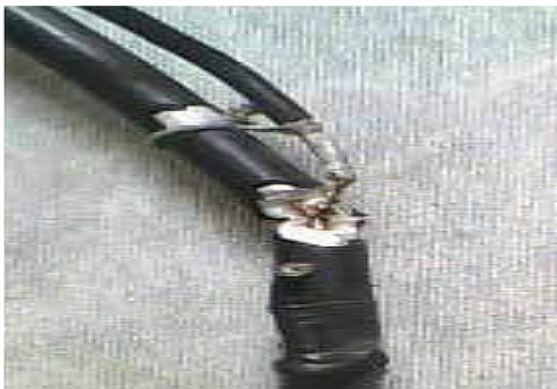
Damaged Cable due to Illegal connection could cause reflections
